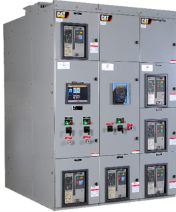
Figure 2 Cat paralleling switchgear with integrated controls and switchgear featuring color touchscreen operator interface.
